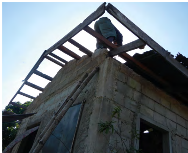
Roof repairs commence on one house in the Cebu shelter project. ©Norfil
