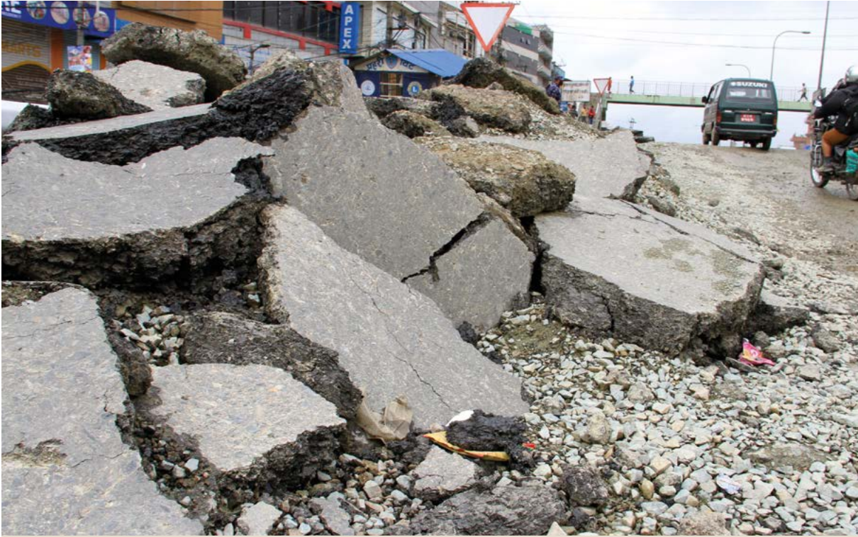
Damaged infrastructure can create extra barriers to accessing relief. ©CBM
