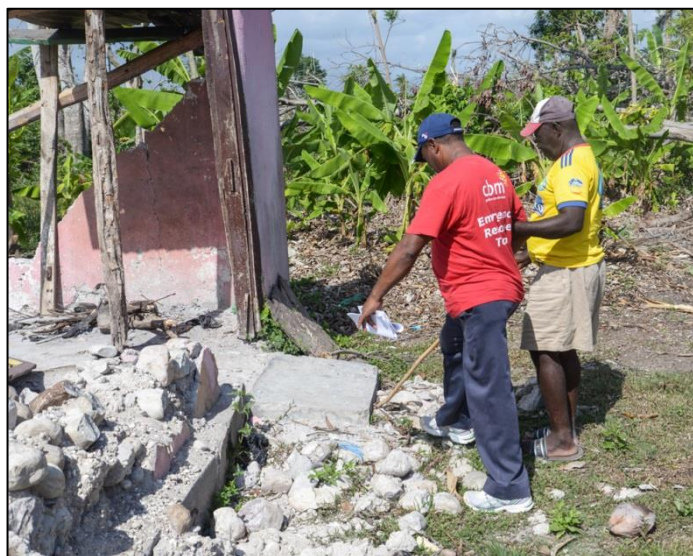
Renee showing CBM Community Worker Homer Auguste what is left of his house after Hurricane Matthew made landfall ©CBM/Abraham
